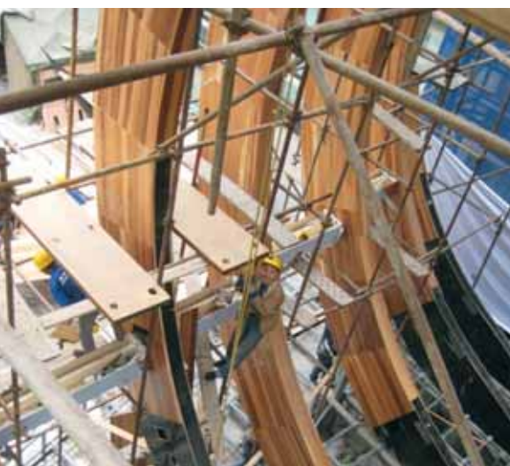
Workers help construct the 13 arches outside the B.C. Canada Pavilion in Beijing, China
